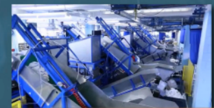
SORTING AND BAGGING LAUNDRY SYSTEM
